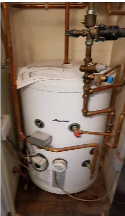
Boiler well maintained and located away from classrooms
