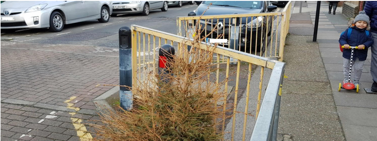
Raised build-outs too short and vehicles park too close or over build out areas
