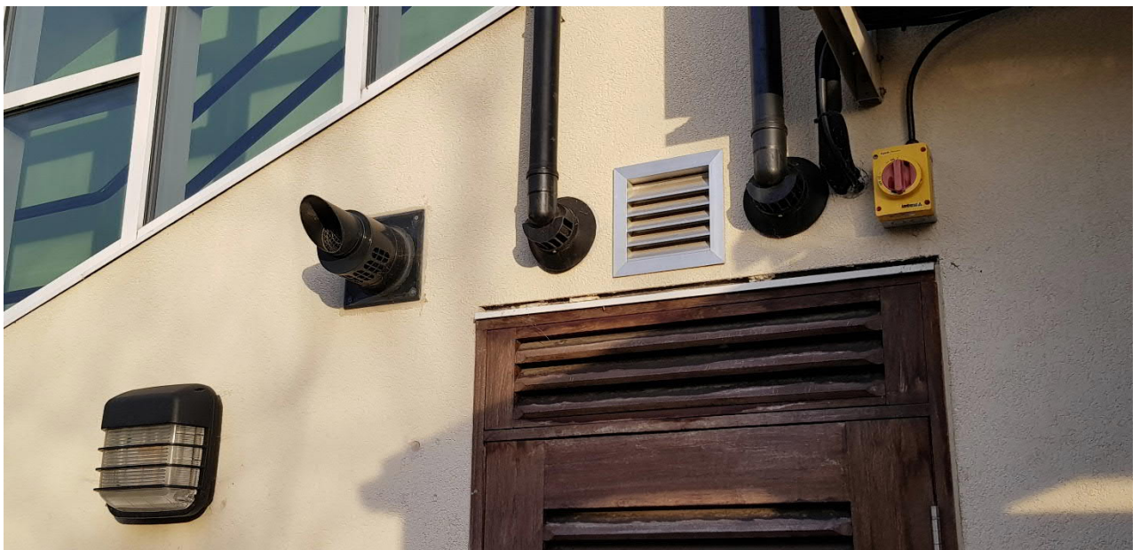
Boiler flues protrude into playground but have been extended upwards
