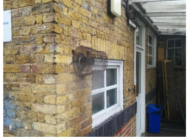
Example flue that discharges at wall height
