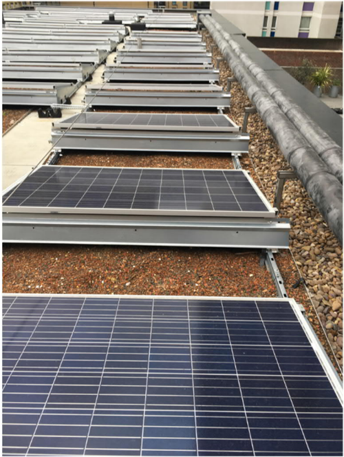
Photovoltaics on the nursery roof
