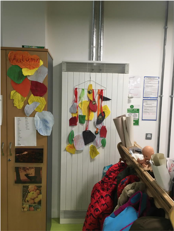
Radiator in Over 3's classroom
