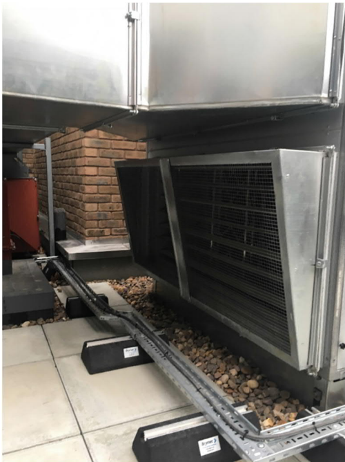
Air Handling Units with HEPA filters
