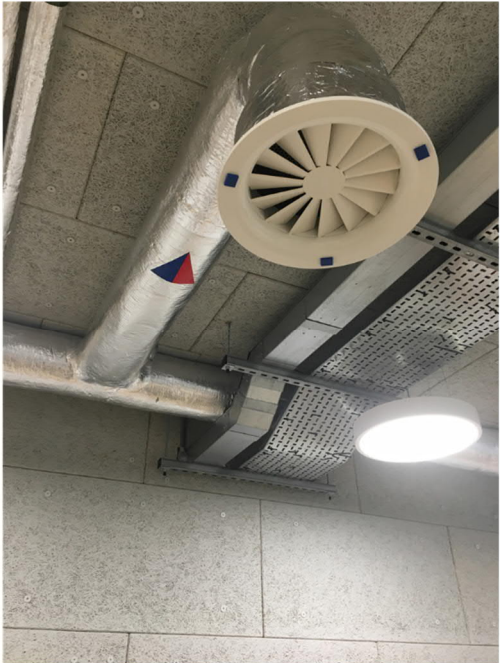
Centralised mechanical ventilation throughout the building
