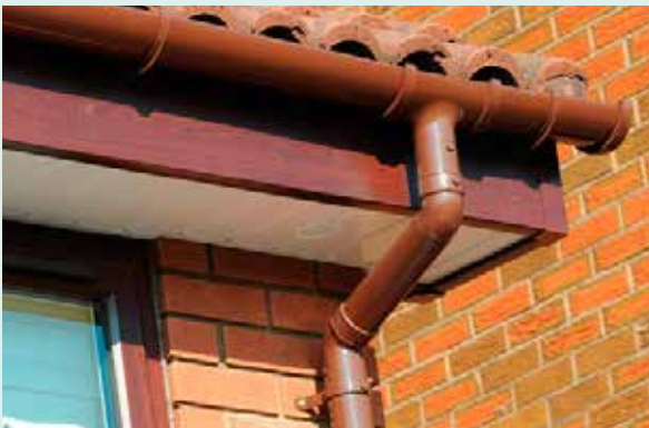
Rainwater pipe not considered in design of facade as a whole
