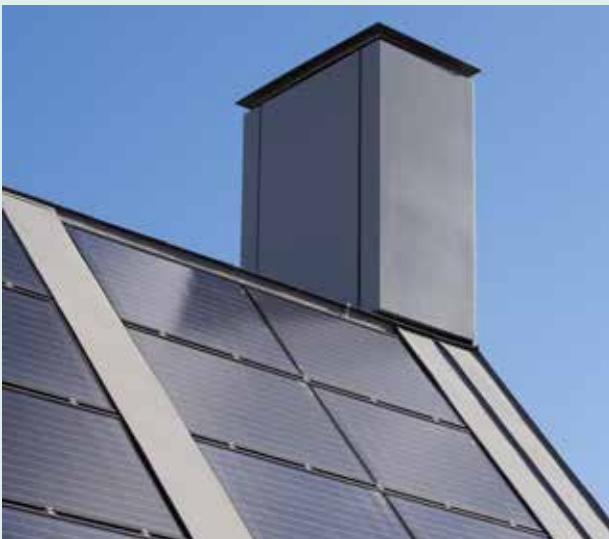
Services to roof are considered and incorporated in a way which enhances the overall roofscape
