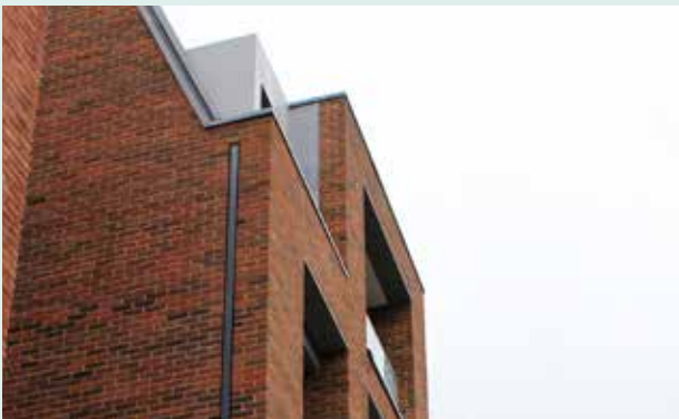
Recessed rainwater pipe
